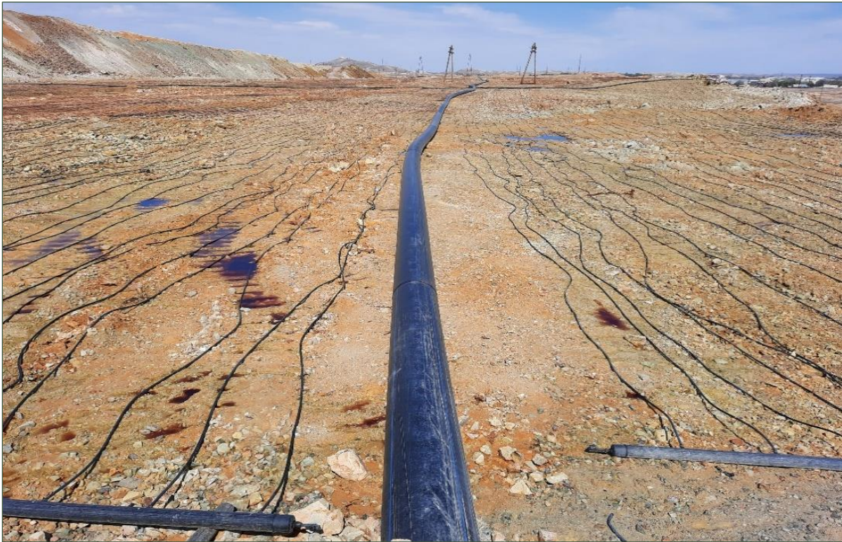
Figure 16-2: Dump Leaching Dripper System
